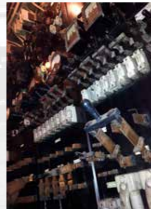
Electrical switch gear
